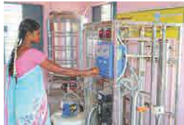
Community RO plant at Malaipattu village, Kancheepuram
